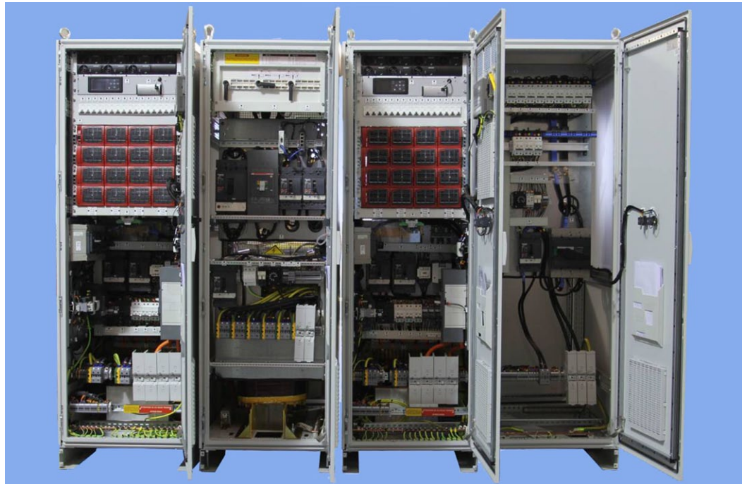
Fig. 1: The two inverter cabinets each contain 16 TSI BRAVO EPC 110Vdc/230Vac Inverters, in EPC mode. Each inverter module has an output of 2.5kVa, making 40kVa in total.
